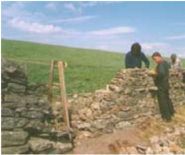
A side wall of stone being built, note the stones going through the wall
