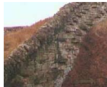
The stones going through the wall are known as tiebands, through stones or thrusts.
