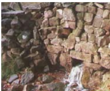
A small hole at the base of the stone wall to let water pass through is known as a "Water Smoot"
