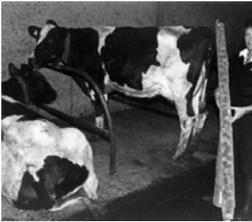
A carpet being laid in the cubicle house for the dairy cows comfort
